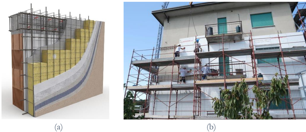
Figure 2.10. “Geniale cappotto sismico” system: (a) components and (b) application to a residential building located in Treviso (Northern Italy) [35]
