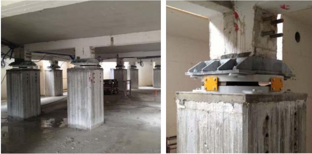
Figure 2.5. Retrofit intervention by means of seismic insulation technique in a residential building located in the city of L’Aquila (Central Italy) [18]
